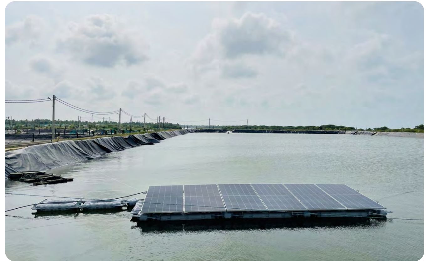
Floating Solar Pilot Project at Taprobane Shrimp Farm Erukalampidy, Mannar
